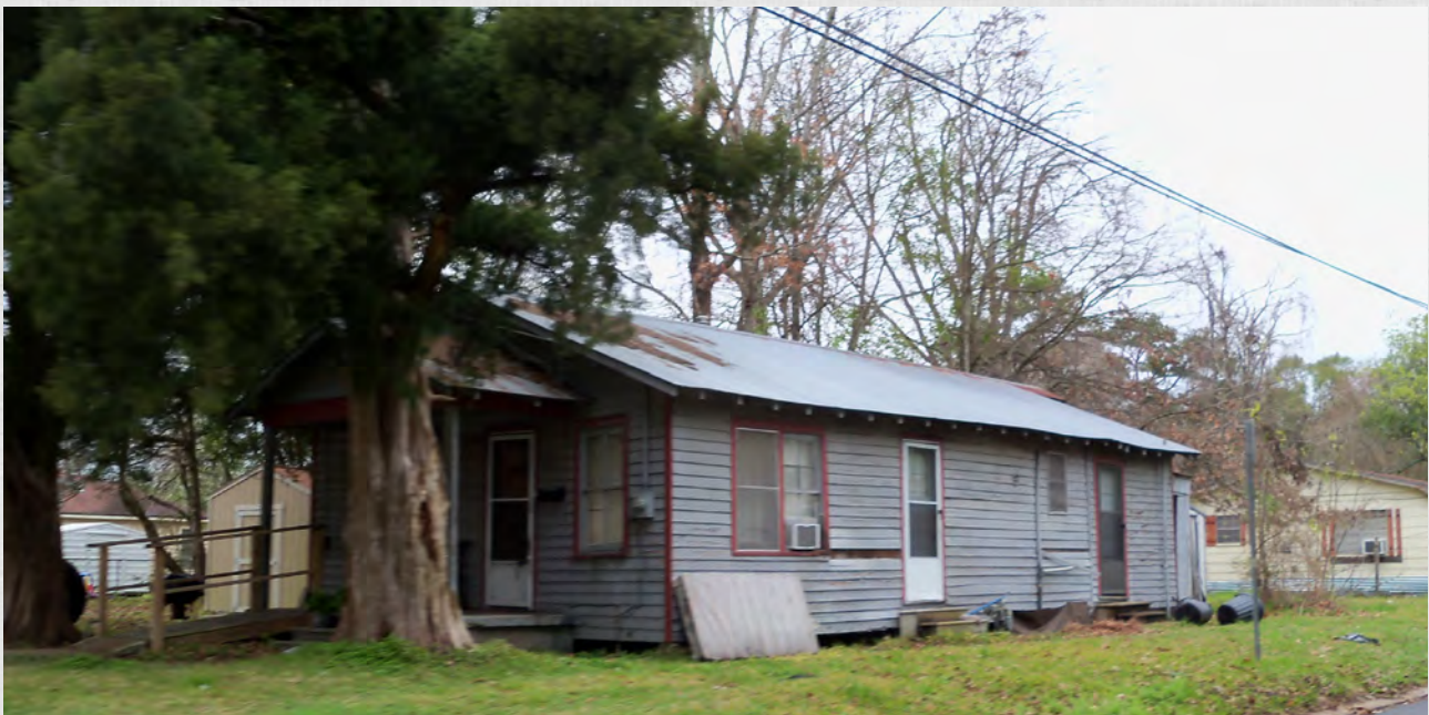
Simcoe Street: Housing in need of repair
